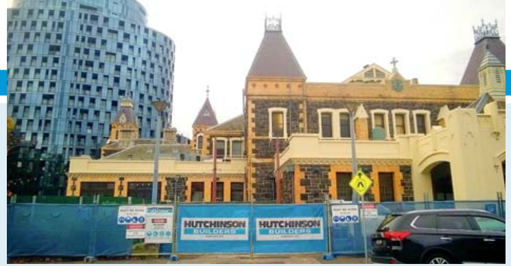
Hutchies is undertaking extensive refurbishment and conservation works to the heritage-listed Royal Victorian Institute for the Blind.
