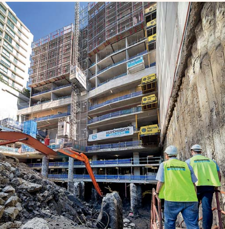
Work goes on above and below ground level with Top Down Construction.
